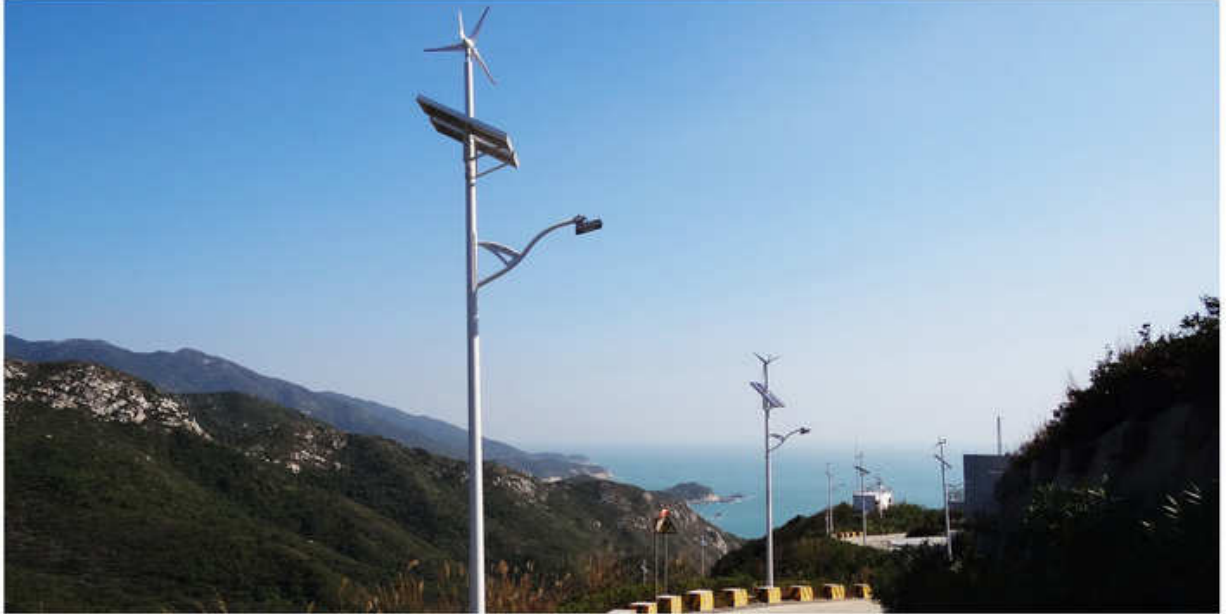
Wind Solar Street Light in Shenzhen
